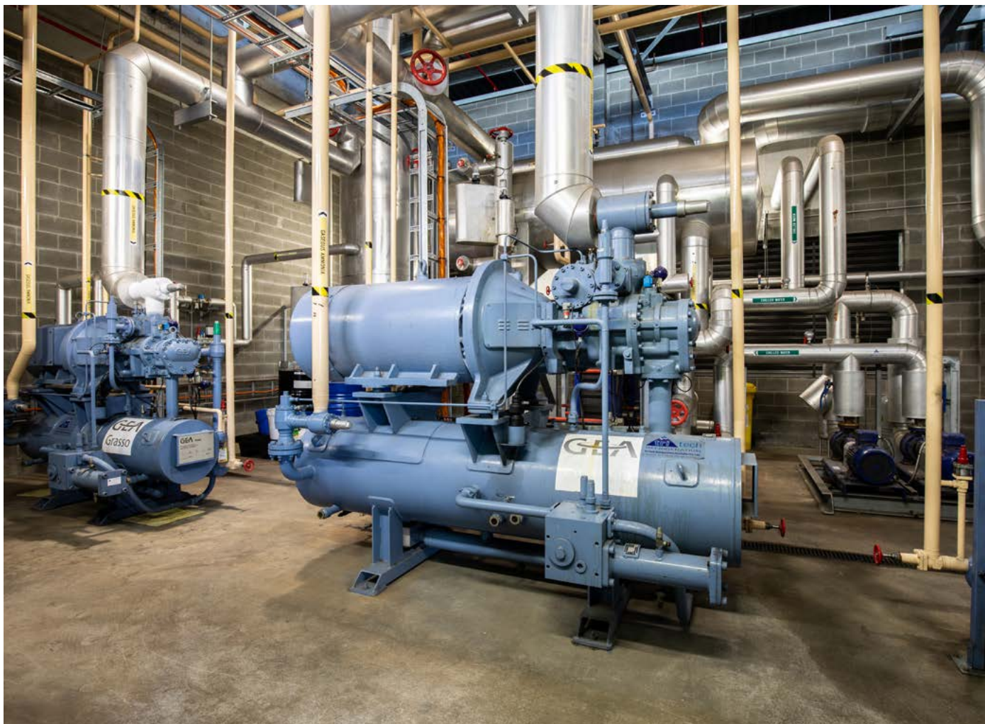
Plant room with ammonia pumped recirculation and water chiller compressor packages.
